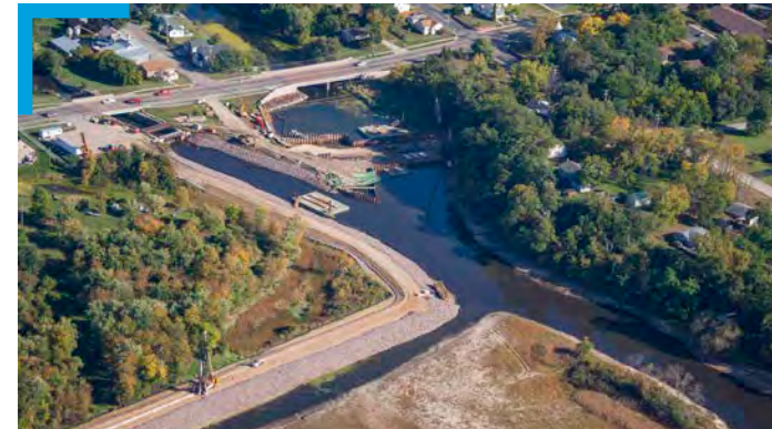
Montello Dam Reconstruction Montello, Wisconsin Reconstruction of the embankment and spillway with a vibrating beam slurry wall to increase stability and reduce the risk of failure
