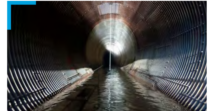
Broken Bow Dam Diversion Tunnel Broken Bow, Oklahoma Analysis of the structure condition, stability, and electrical and mechanical components of concrete-lined diversion tunnel
