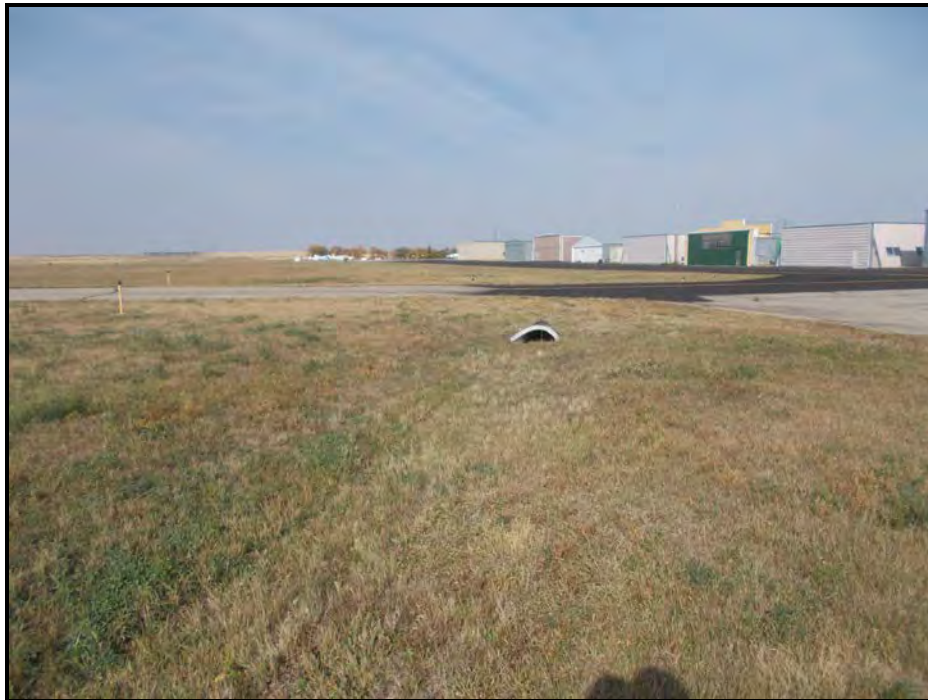
Photograph 2. View of Ephemeral Drain 1b taken facing northwest. The constructed drain conveys water away from the airport into Wetland 1a.
