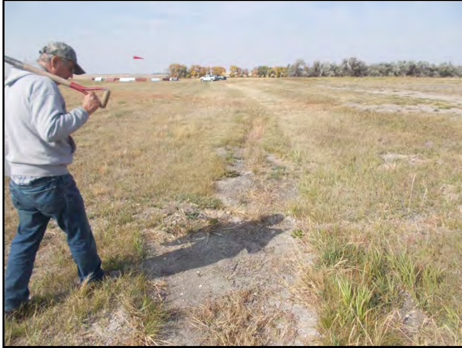
Photograph 5. View of Ephemeral Drain 3a taken facing west. The constructed drain conveys water from the Airport Facilities to the west and away from the hangers. The constructed drain is well vegetated with slender wheatgrass. Observation Point 30 was evaluated within the drain near the vehicles in the background off the photograph.
