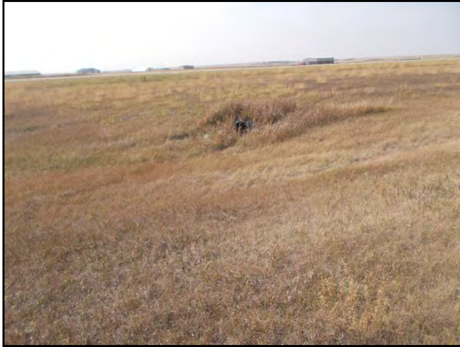
Photograph 7. View of culvert that flows storm water south under the runway and into Ephemeral Drain 5a. Photograph taken facing south. Ephemeral Drain 5a conveys water south and under 61 st Street. Observation Point 32 was evaluated near the culvert location.
