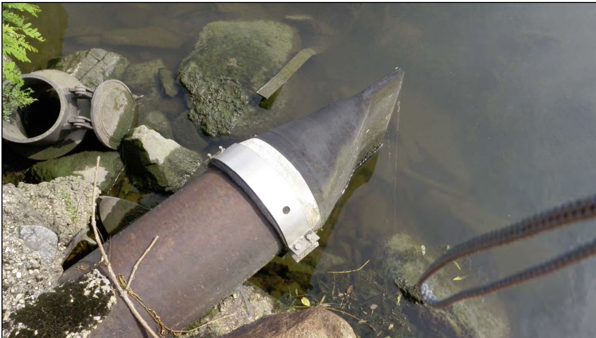
Figure 4.7: Typical Existing Duckbill Valve in Port Deposit
