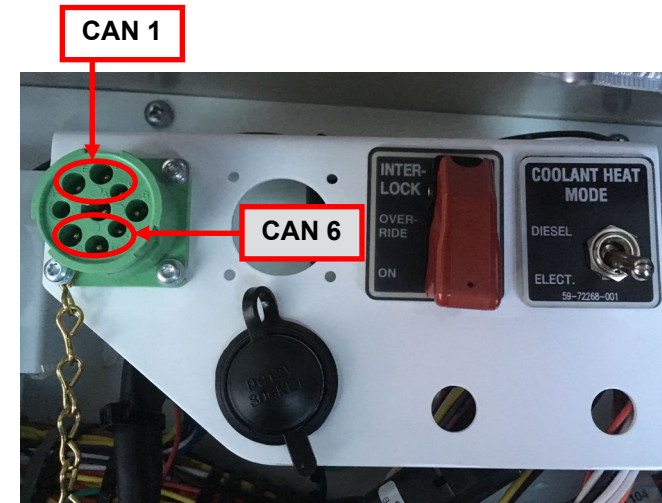
Front Electrical Panel
