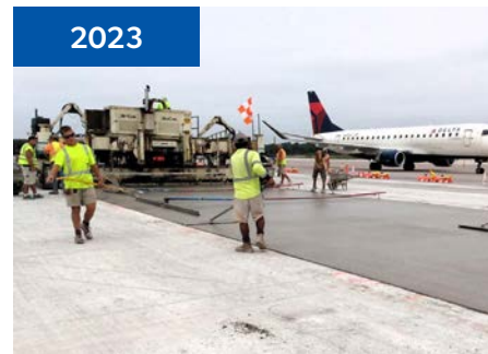
2023 Green Bay Austin Straubel International Airport Taxiway and Apron Rehabilitation Wisconsin Bureau of Aeronautics Outstanding Airport Construction Project
