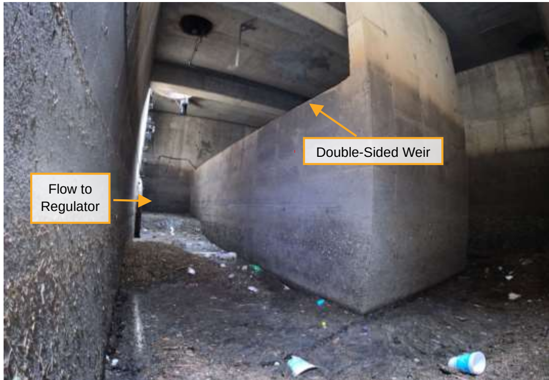
Figure 42 | Spring Regulator, Influent Side of Structure
