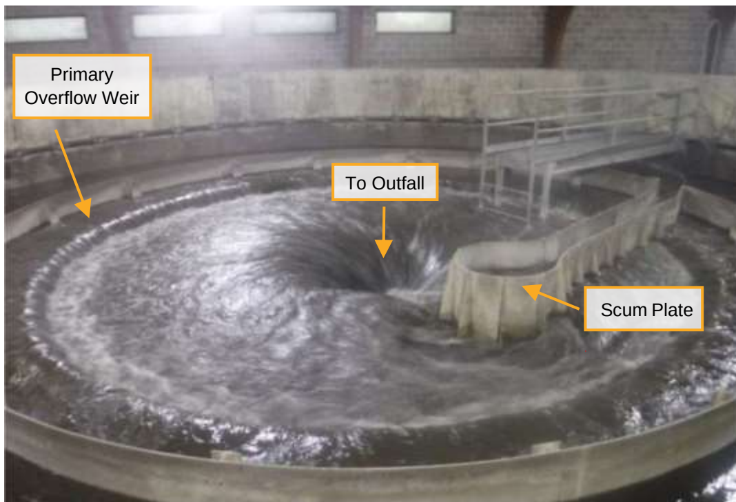
Figure 35 | Eaton Swirl Concentrator, from Above During Active Overflow
