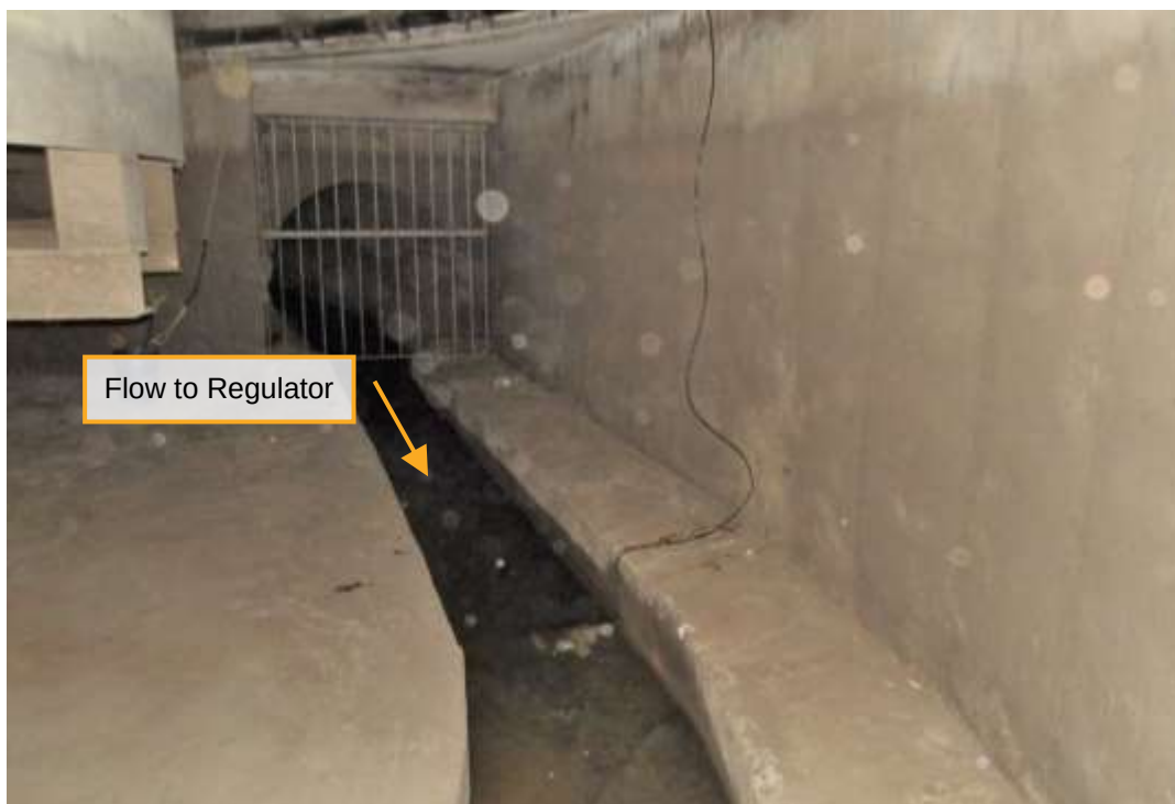
Figure 36 | Eaton Swirl Concentrator, from Downstream Looking Upstream at Influent Pipe
