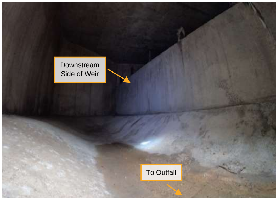
Figure 31 | Fayette Regulator, from Overflow Side of Weir
