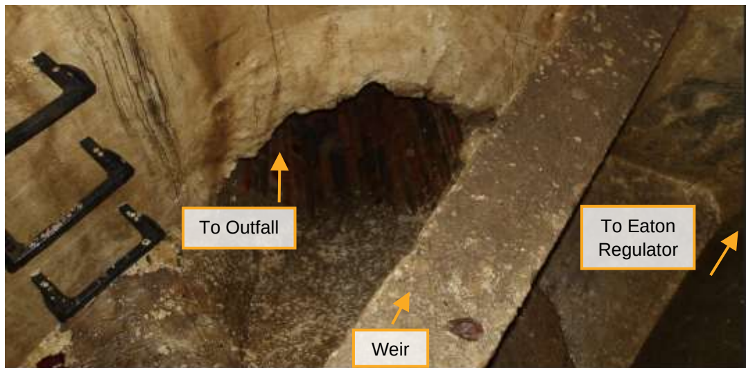
Figure 41 | Green Regulator, from Above Showing Outfall Pipe
