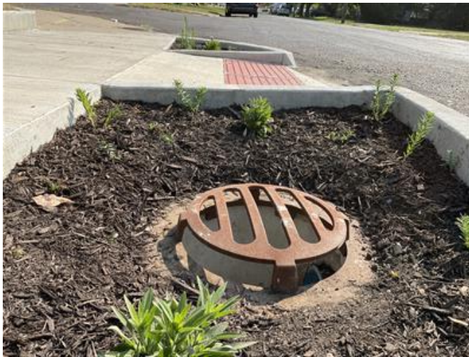
Figure 6 | Showing Inlets in Stormwater Bump Outs in Year 1 Project Area. Photos taken August 29, 2023.
