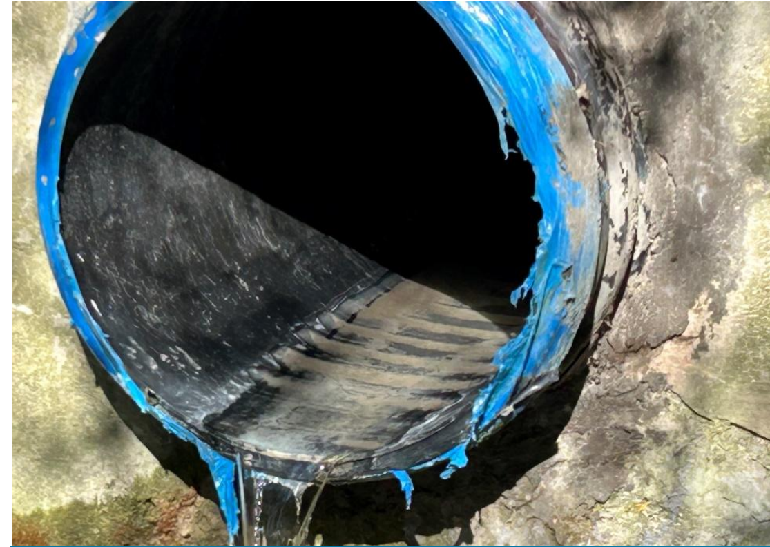
Outfall from PPSD 150 Illicit Discharge
