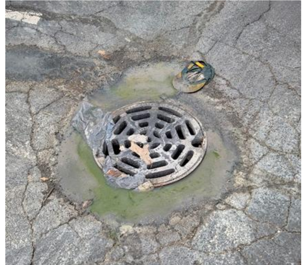
Peoria Grease Trap Spill
