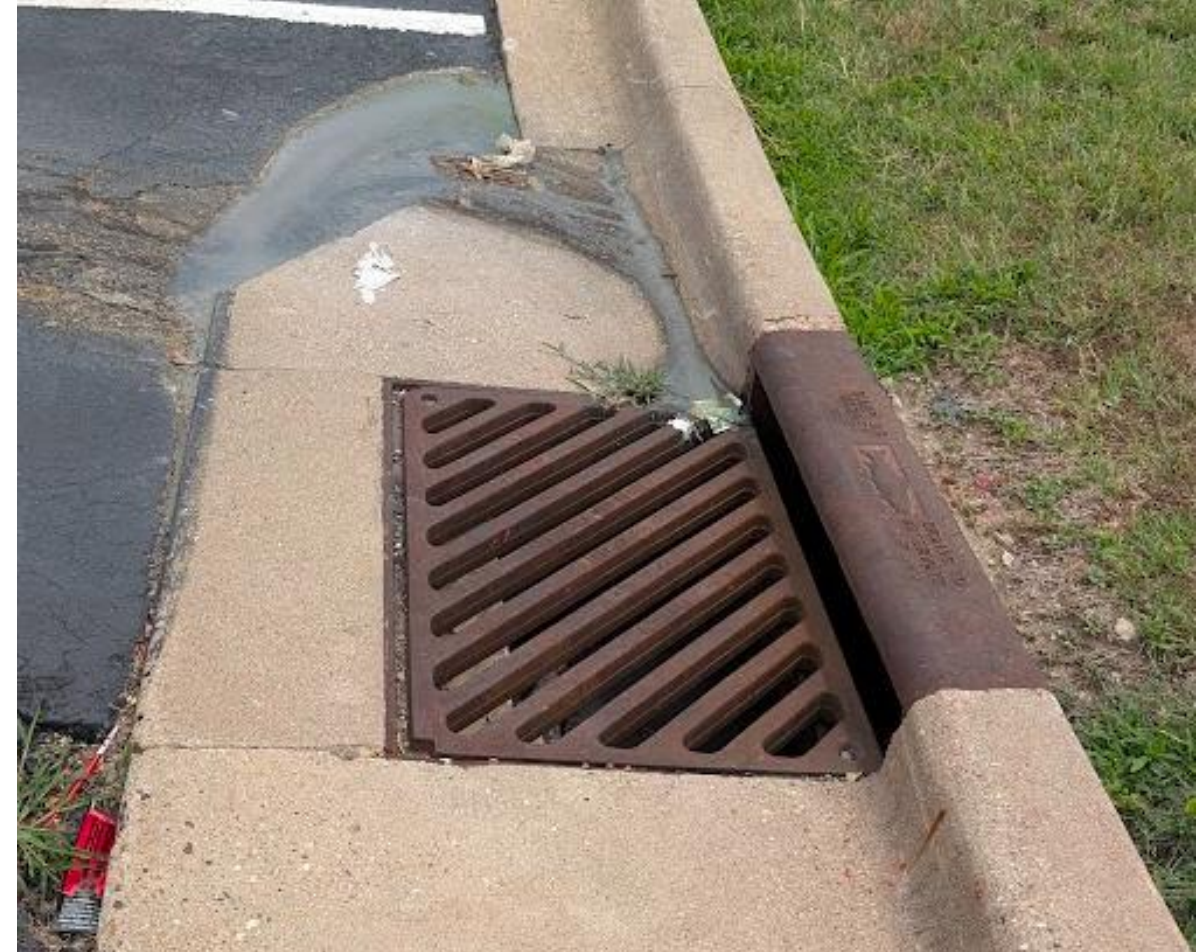
Grease Trap Spill
