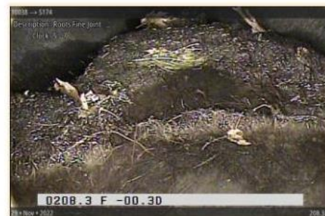
[Grade 1] Roots Fine Joint at 208.3 ft, 5 - 7 o'clock
