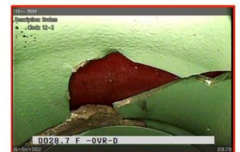
[Grade 4] Broken at 028.7 ft, 12 - 2 o'clock
