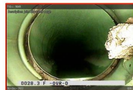
[Grade 4] Joint Separated Large at 028.3 ft
