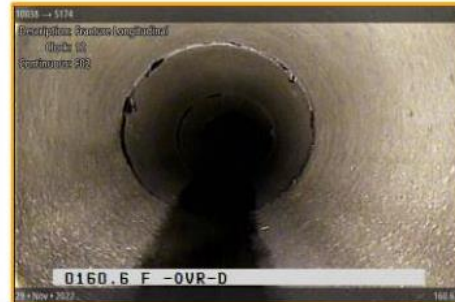
[Grade 3] Fracture Longitudinal (finish) at 160.6 ft, 12 o'clock
