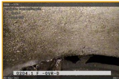
[Grade 3] Roots Medium Joint at 204.1 ft, 8 o'clock
