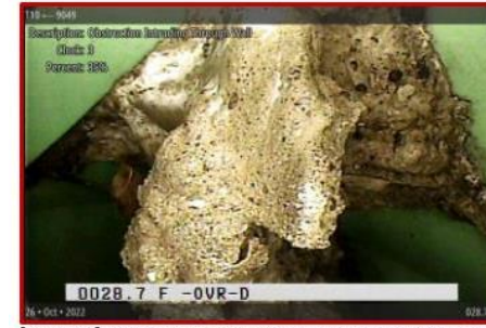
[Grade 5] Obstruction Intruding Through Wall at 028.7 ft, 3 o'clock
