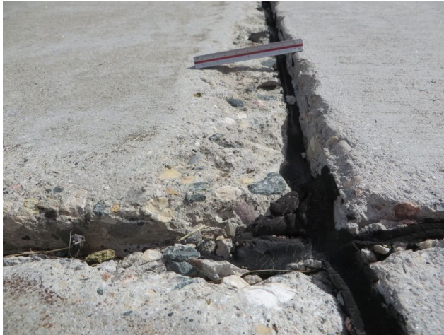
Faulting on Taxiway Connector
