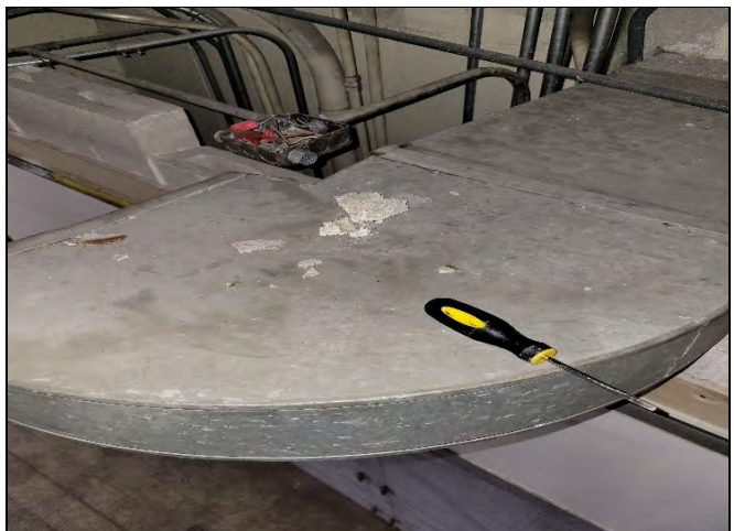
Asbestos Insulation Debris on Ductwork, NE side Behind Restroom
