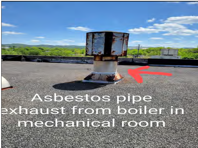
Asbestos Cementitious pipe as boiler flue, Mech Room to Roof
