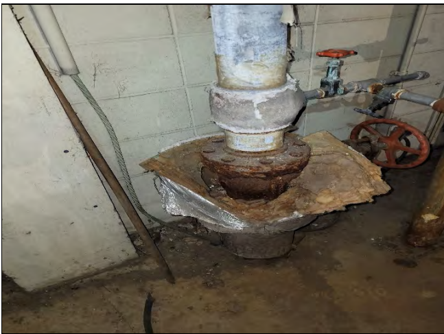
Asbestos Insulation covering Valve, Mechanical Room
