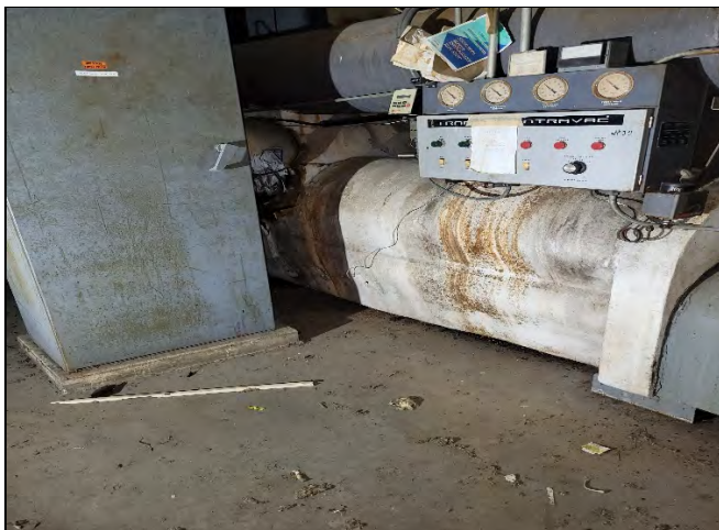
Asbestos Insulation on Chiller in Mechanical Room
