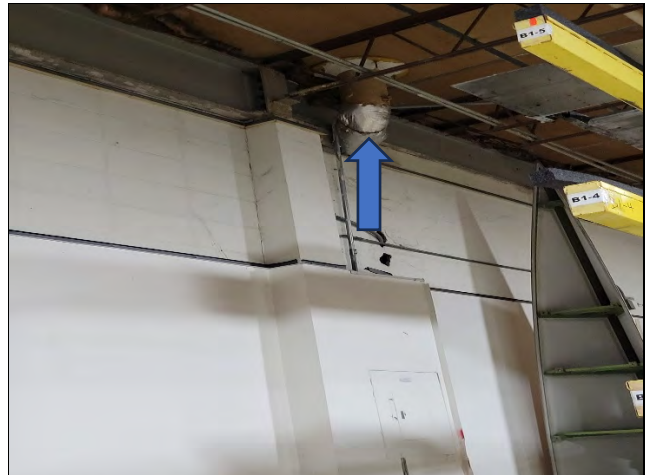
Asbestos Insulation on Drainpipe Elbow, SW Corner
