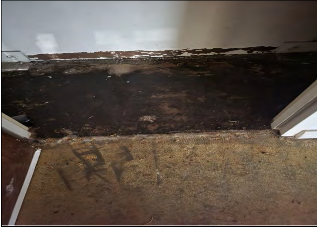
Asbestos Black Mastic on Concrete in Closet, Room W-4
