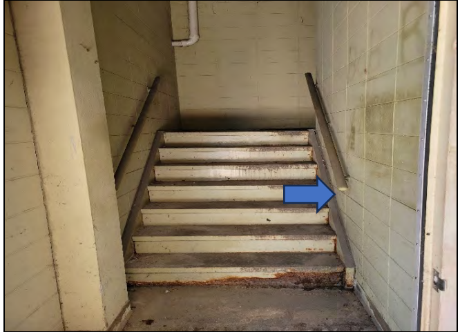
Asbestos Caulking between Wall and Stairs
