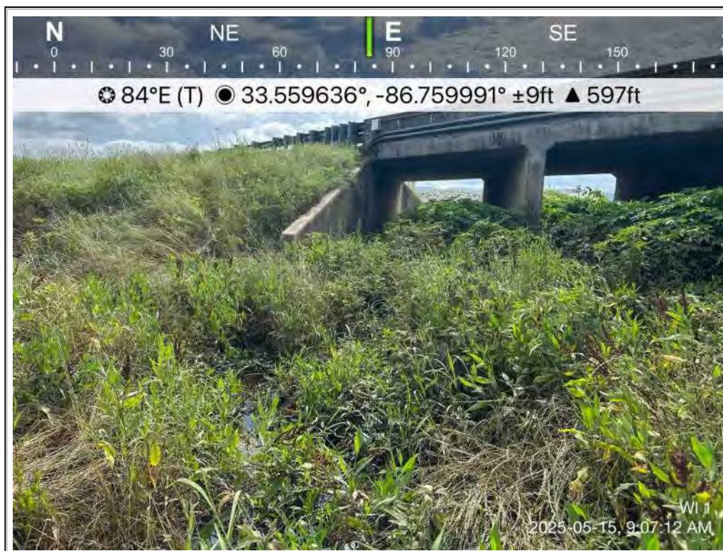
Picture 2: View of WL2
