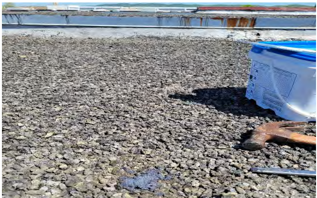
Asbestos Flashing and Asbestos Black Mastic, Parapet Wall
