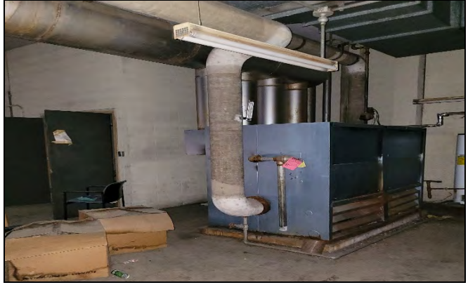
Asbestos Insulation on large Pipe Elbow, Mechanical Room
