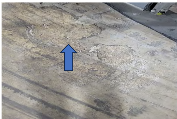
Asbestos 12"x12" Floor Tile Over Asbestos Black Mastic, NE Center, Main Area
