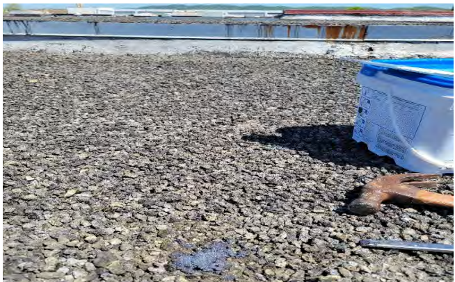
Asbestos Flashing and Asbestos Black Mastic, Parapet Wall
