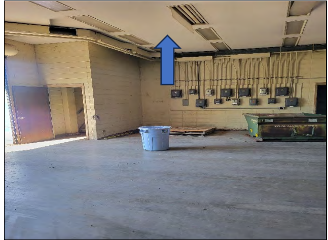
Wallboard Ceiling with Asbestos Joint Compound, SW
