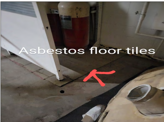
Asbestos 9"x9" gray FT and Asbestos Black Mastic, SE corner outside Computer Room
