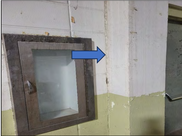
Asbestos Caulking at Joint between Column and Wall, NW Corner
