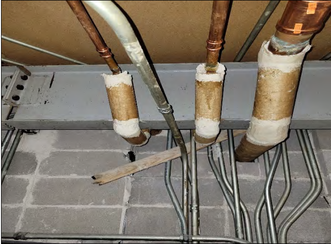
Asbestos Insulation on Pipe Elbows-Damage Areas, Main Area behind East Side Restrooms
